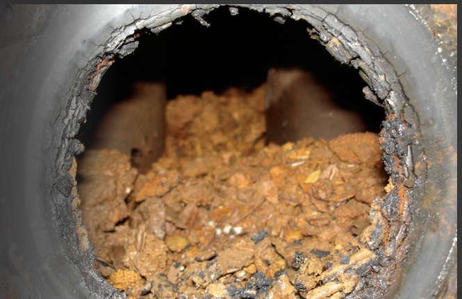
"In-tank" flue tubes and heat exchangers suffer from lime scale buildup beginning from the first hours of operation.
